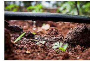
Inline Drip system
